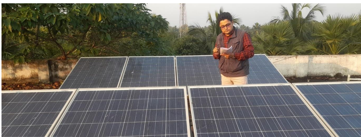
Solar Energy module of Ramnagar College
