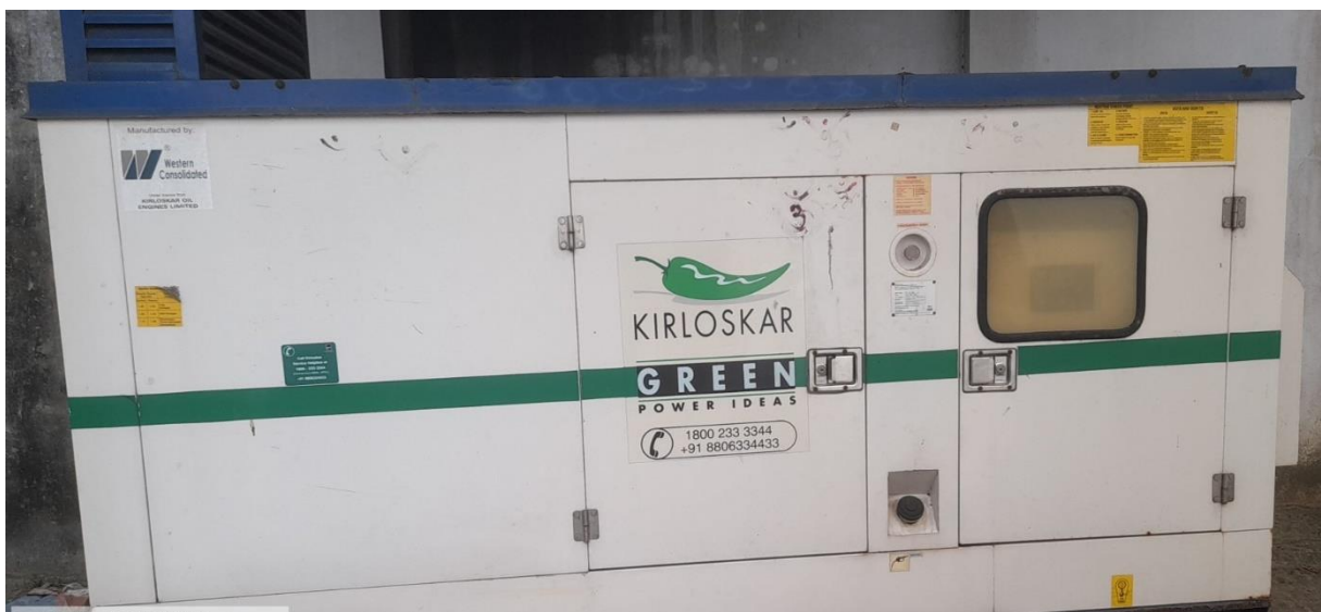
Emergency supply line at Ramnagar College
